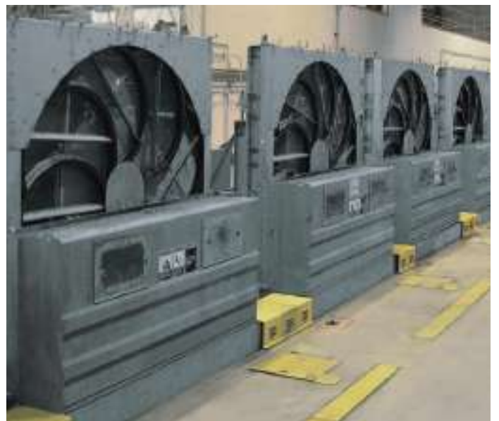
DC Cook Nuclear Power Plant, USA
