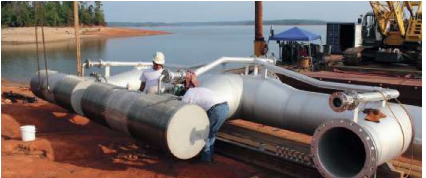
Johnson Screens® Passive Intake Installation: Drinking Water Plant, in South Carolina, USA
